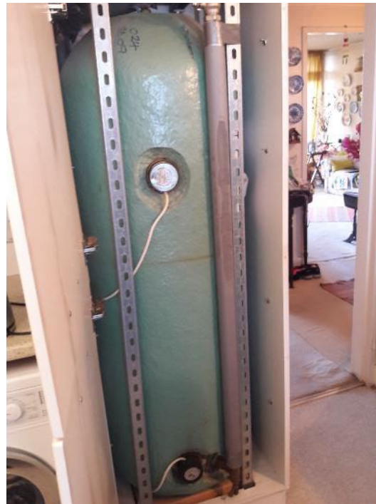
Hot Water Cylinder
