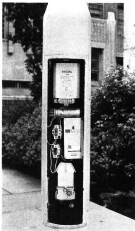
Cyclocontrol receiver installed in lamp standard
